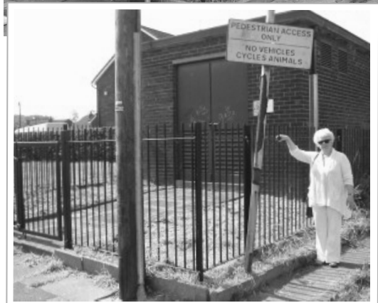
One of the Ward's sub-stations before and after the clean-up
